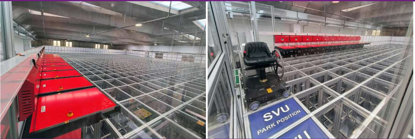
Dematic has successfully installed an AutoStore™ automation system for Plurima (Photo: Dematic)
